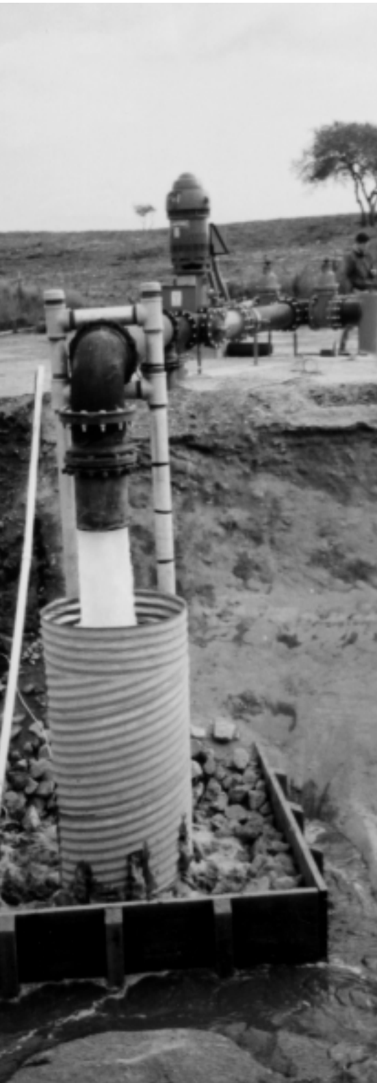
MPWMD staff conducting well “backflushing” at the test injection well. During backflushing, water from the well is pumped to an adjacent settling basin at up to 3,000 gallons per minute (gpm) to free up fine particles that can get swept into the well during injection.
