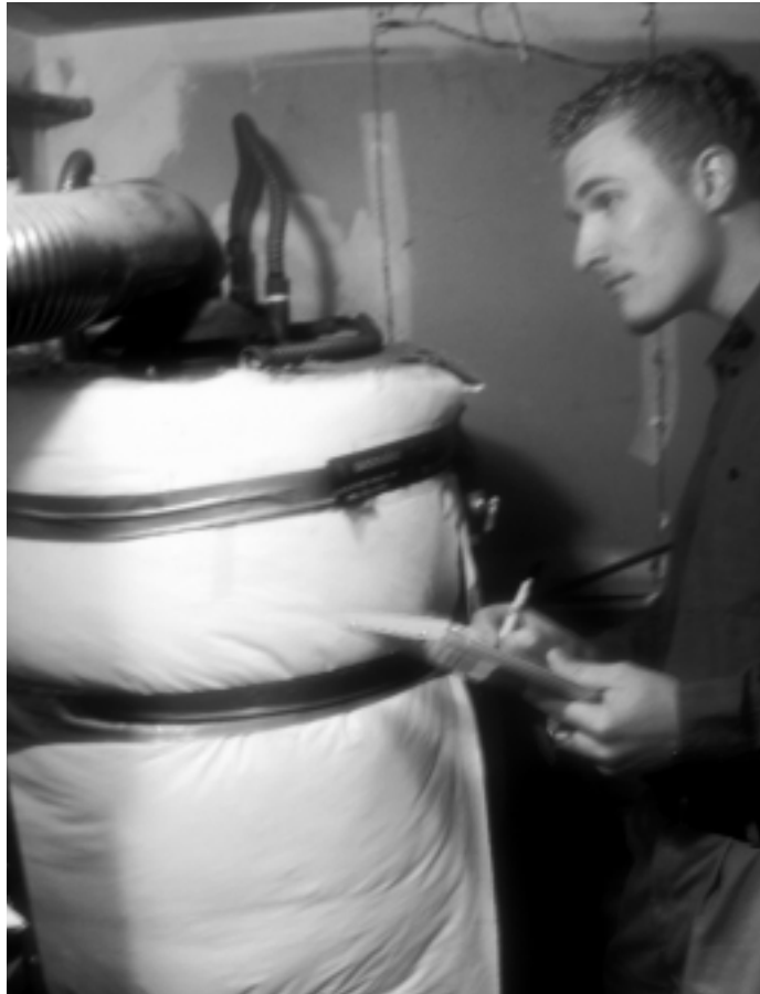
Rob Cline, MPWMD, inspects a water heater in a Pacific Grove apartment building, as part of the District's conservation monitoring.
