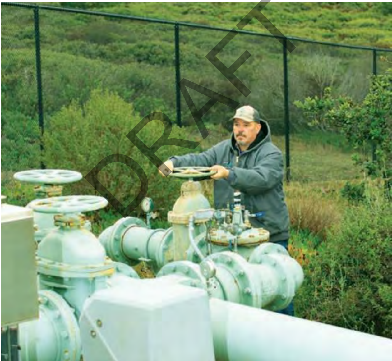
(Photo: (ASR) Aquifer Storage and Recovery Project)
